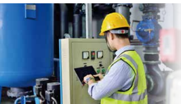
Control panels at industrial plants
