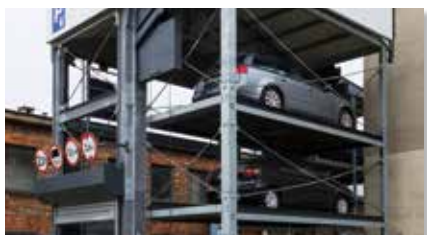
Maintain automated car parking systems
